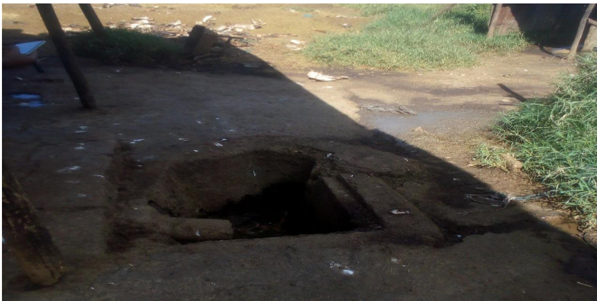
Photo 6: Liquid waste disposal pipeline
